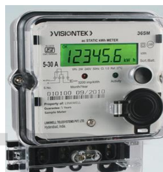
Fig 2. Electronic power meters
